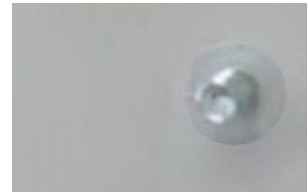
Fig. 20: Unmarked grounding stud
