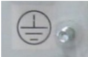
Fig. 19: Grounding stud marked with PE symbol
